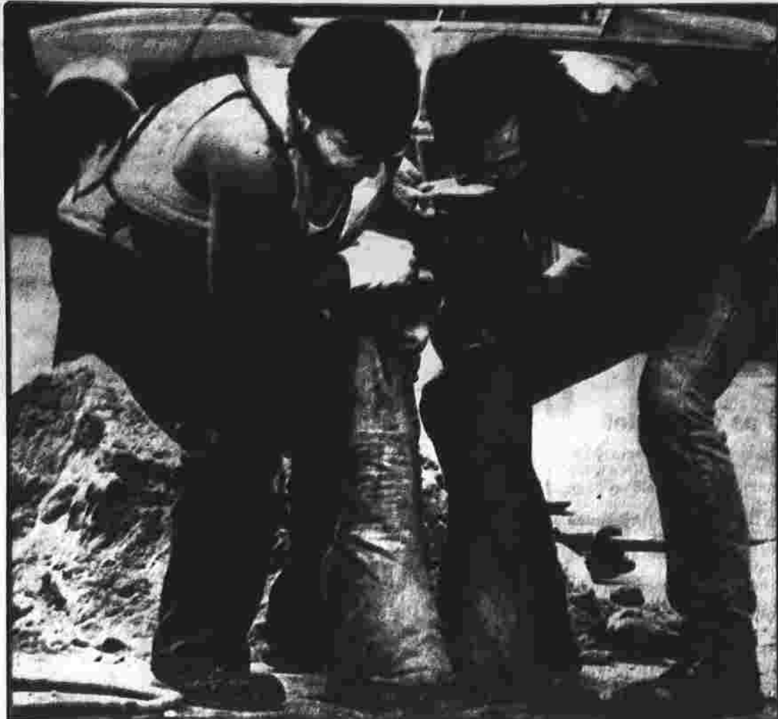
Leonard Boso, left, and Wiley Chen hold onto Rich Chichester as he works through a hole in a road in Concord, N.H., recently. The three men work for a firm doing preventive maintenance for Concord Natural Gas Corp.
